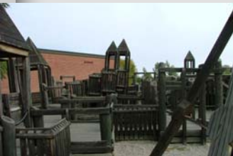
Current elementary playground. Notice the shifting of the structure that has taken place.
